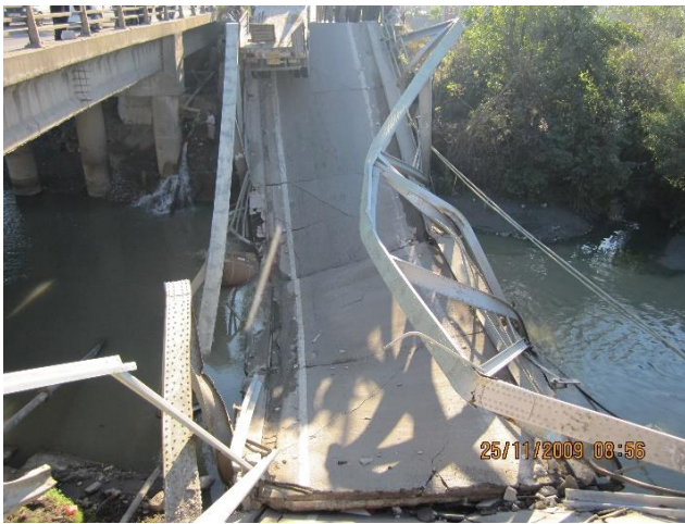
Fig. 2. the collapse of Sardabroud bridge due to heavy load collision with a key element of the structure
